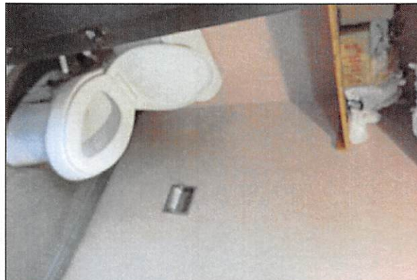
Employee bath in kitchen bay
