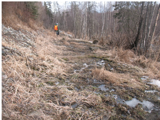
Leakage at Toe of Percolation Bed 6
