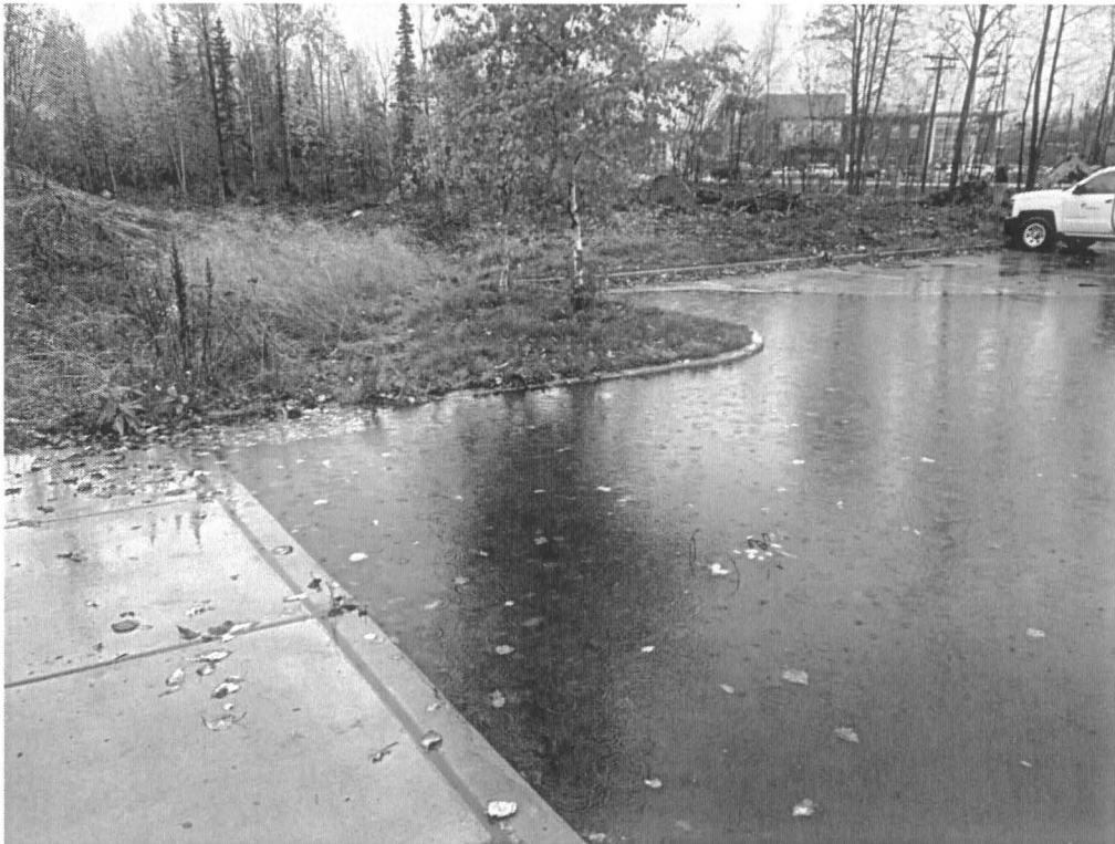
Water ponded in northwest corner of existing parking lot.
