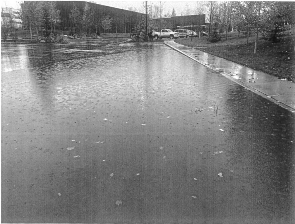
Water ponded in northwest of parking lot
