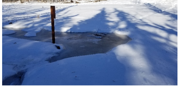
Photo 3: Discharge Bed #1 on Feb. 27
