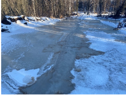
Photo 1: overflow on berm
