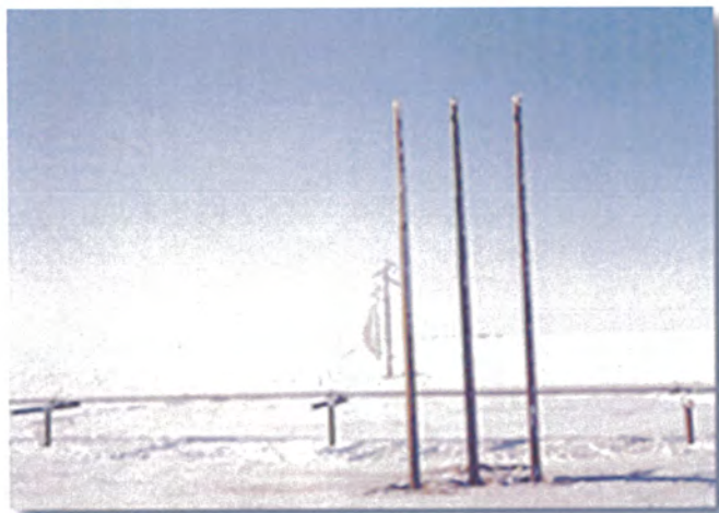
ARCO West Sak/Kuparuk, North Slope 35 kV Wishbone Transmission
