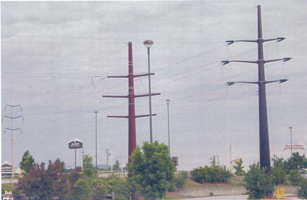
Figure IV-1 - 115kV transmission line structures located near Mall of New Hampshire in Manchester. (Photo by NEI – PSNH System)
