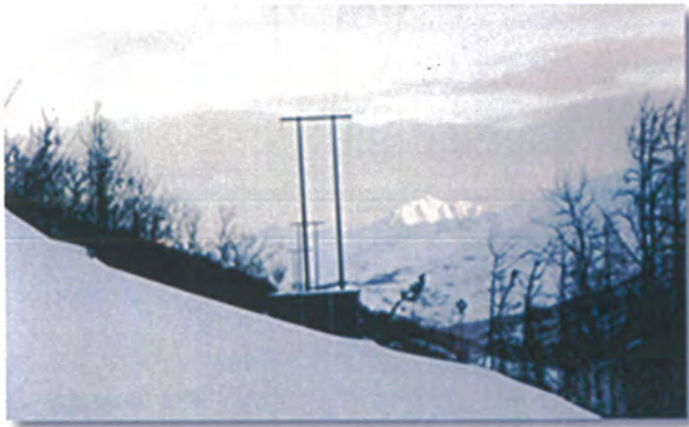
Quartz Creek Line Summit Lake 115 kV Wooden H-Poles Avalanche Diverting Structures
