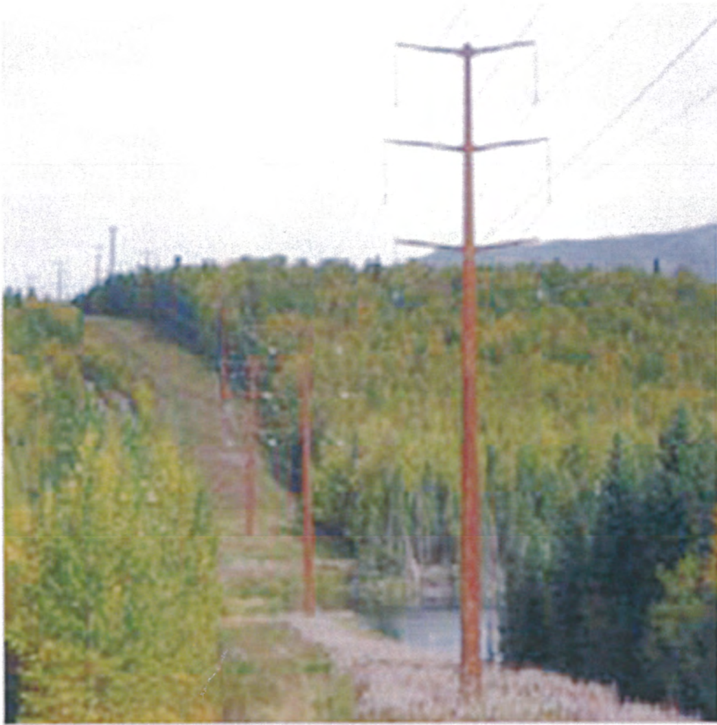
Eklutna Transmission Line 230 kV double circuit on single steel poles
