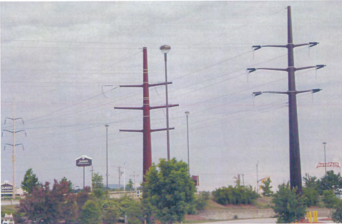
Figure IV-1 - 115kV transmission line structures located near Mall of New Hampshire in Manchester. (Photo by NEI – PSNH System)
