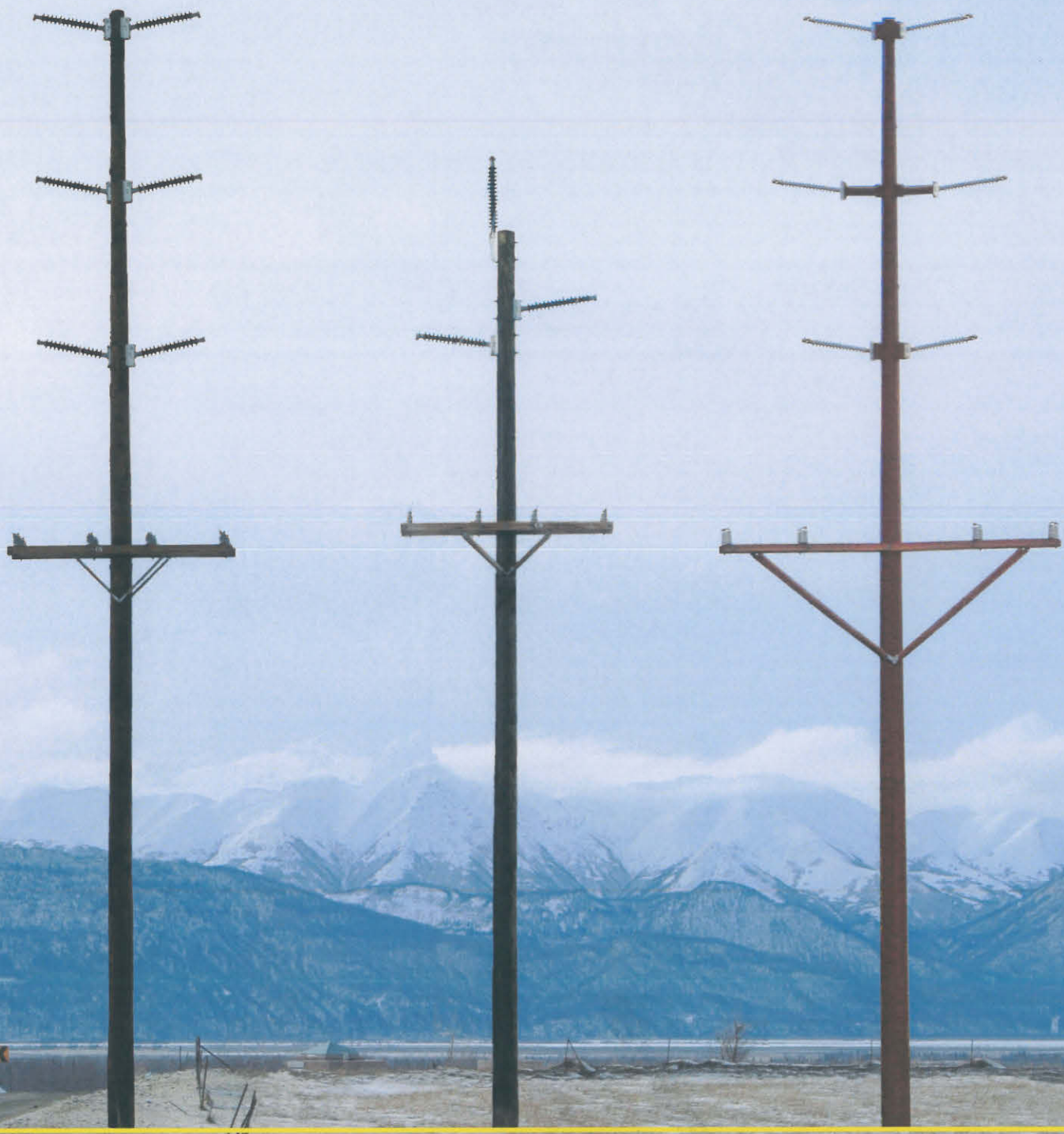
115 kV DOUBLE CIRCUIT: WOOD
